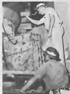
CHECKING THE installation of new skirt plates are R. C. Bergfield and Nasario Tromp. INSPECTANDO INSTALACION ta R. C. Bergfield y N. Tromp.
